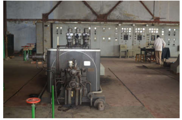
Power turbine+Main Panel Board
